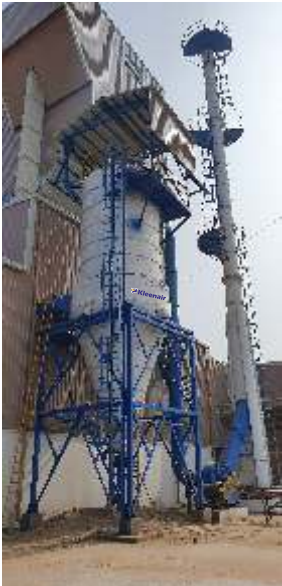
Dryer Debusting System
